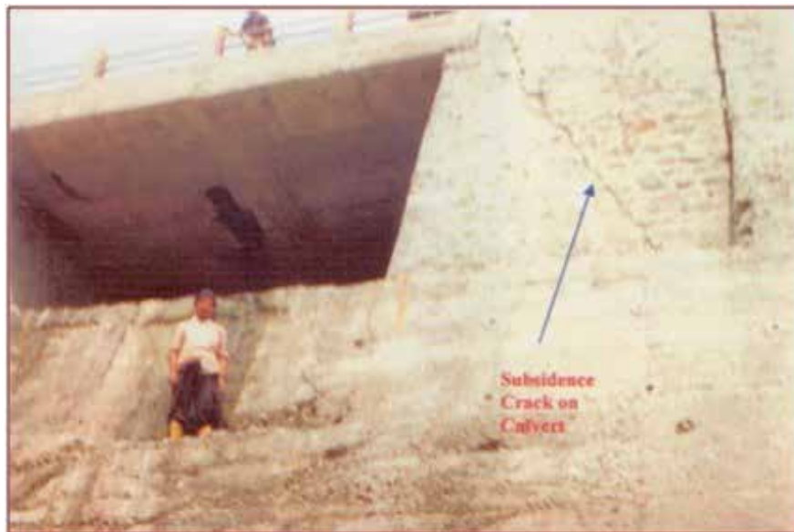
Photograph 4 Subsidence cracks developed on the newly constructed box culvert on the road bench
